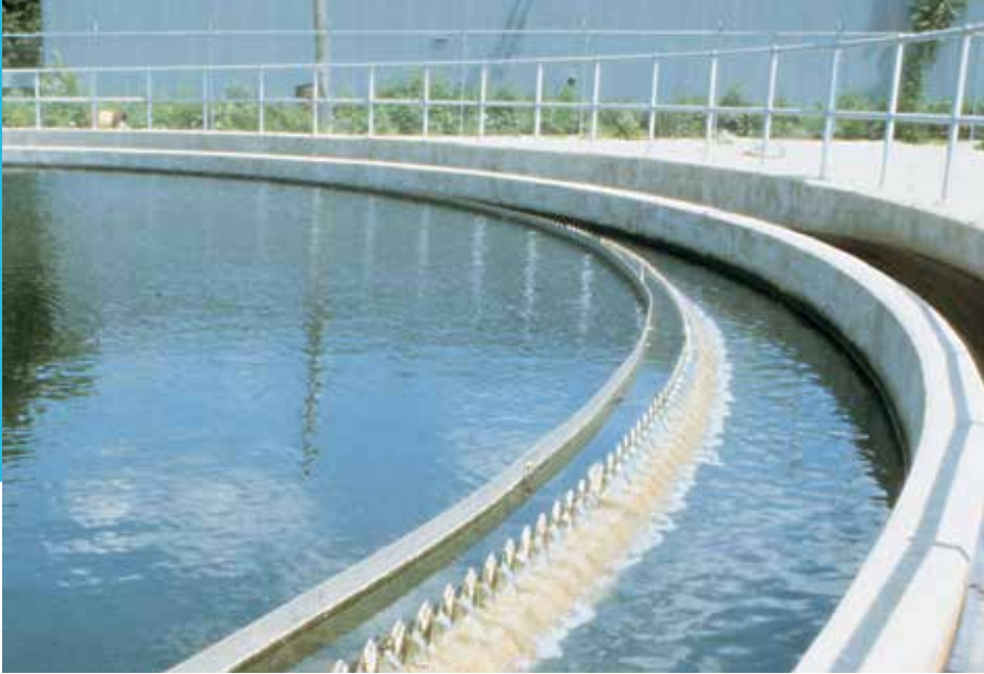
Rim-Flo® system influent and effluent channels
