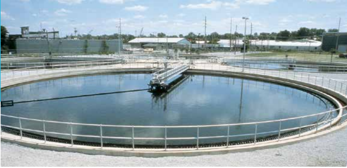
Four 110-foot diameter tanks in this wastewater treatment plant operate at an average raw flow of 400 GPD per square foot of overflow. Effluent BOD ranges from 4 to 6 ppm.
