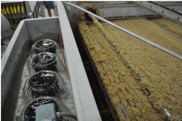
Figure 5. Full-Scale Tertiary DAF Effluent and Float Formation
